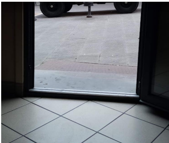
Figure 41 door knocker threshold present at the accessible door
